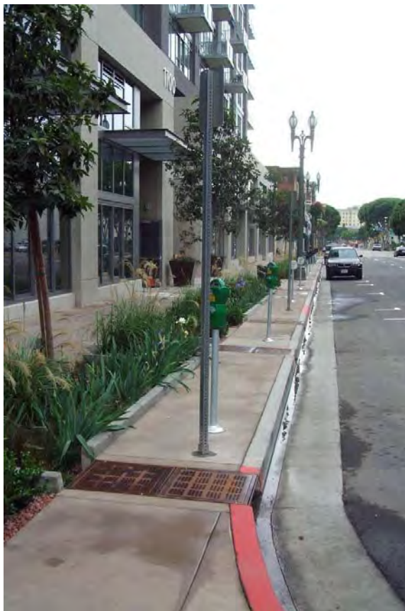
Figure 23. Bioretention cell for street/yard drainage, Los Angeles, CA. Source: Bill DePoto
