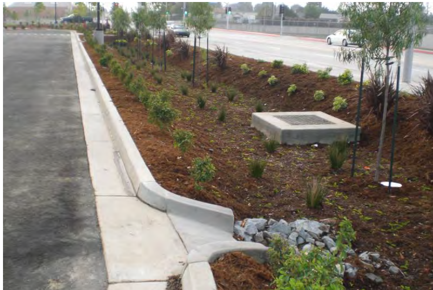
Figure 76. A vegetated swale with curb cuts in El Monte, California. Source: Bill DePoto
