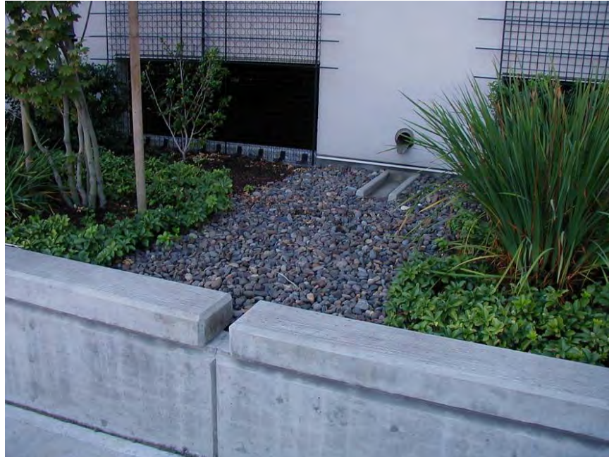
Figure 20. Planter box capturing roof runoff. Source: The Low Impact Development Center, Inc.
