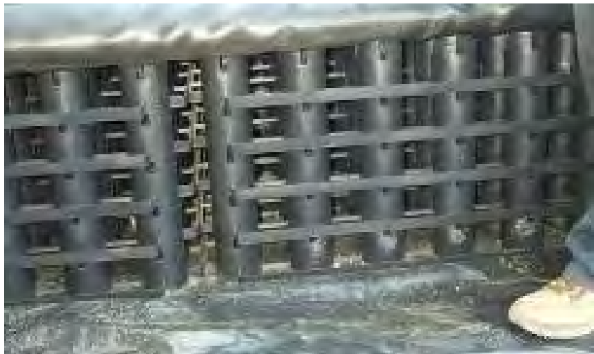
Figure 67. Rainstore™ units used as the storage element underneath a brick pathway atop a vegetated rooftop plaza. Source: Cahill Associates
