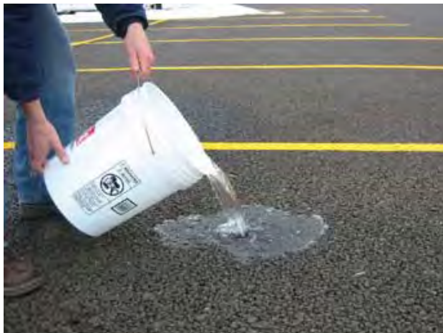
Figure 59. Water on Porous Asphalt. Source: Fishbeck, Thompson, Carr & Huber, Inc.
