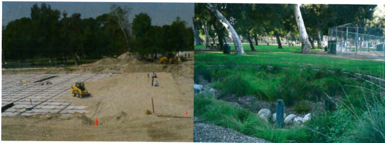
A state-of-the-art Green Solution Project. The Sun Valley Watershed Project uses underground vaults, a surface park, habitat and recreation area to naturally capture and treat polluted runoff from surrounding urban areas. New open space benefits this park-poor community and the project recharges the San Fernando Groundwater Basin, while improving water quality in the L.A. River.
