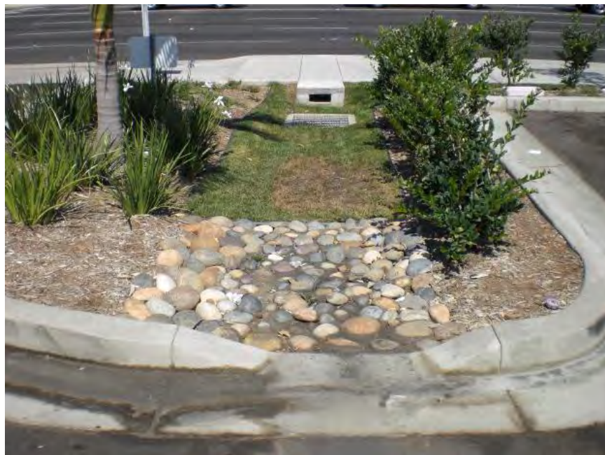
Figure 27. Inlet Structure, Downey, CA. Source: Bill DePoto
