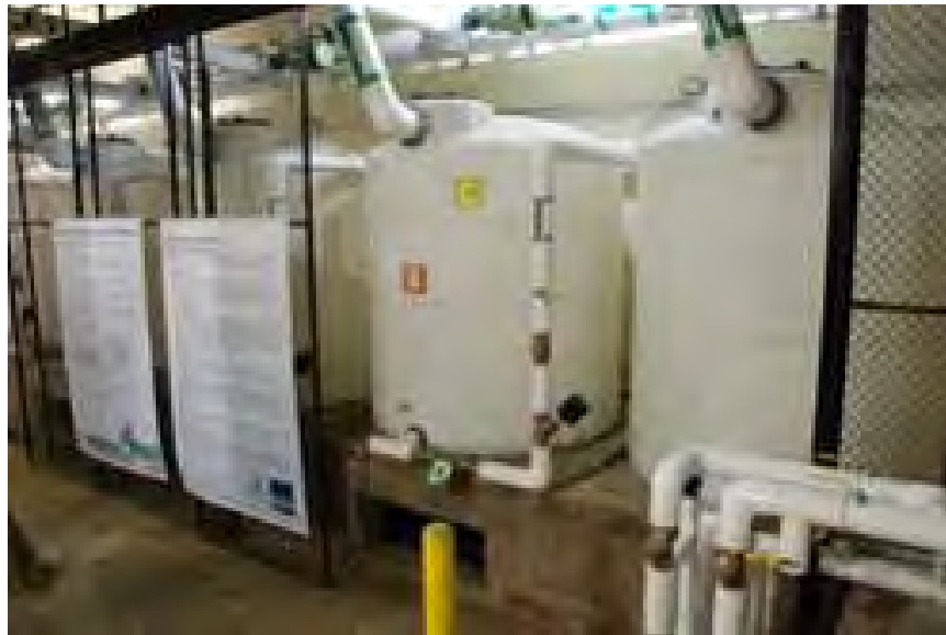
Figure 65. Six (6) 1,000 gallon cisterns at U.S EPA headquarters provide water for irrigation Source: U.S. EPA
