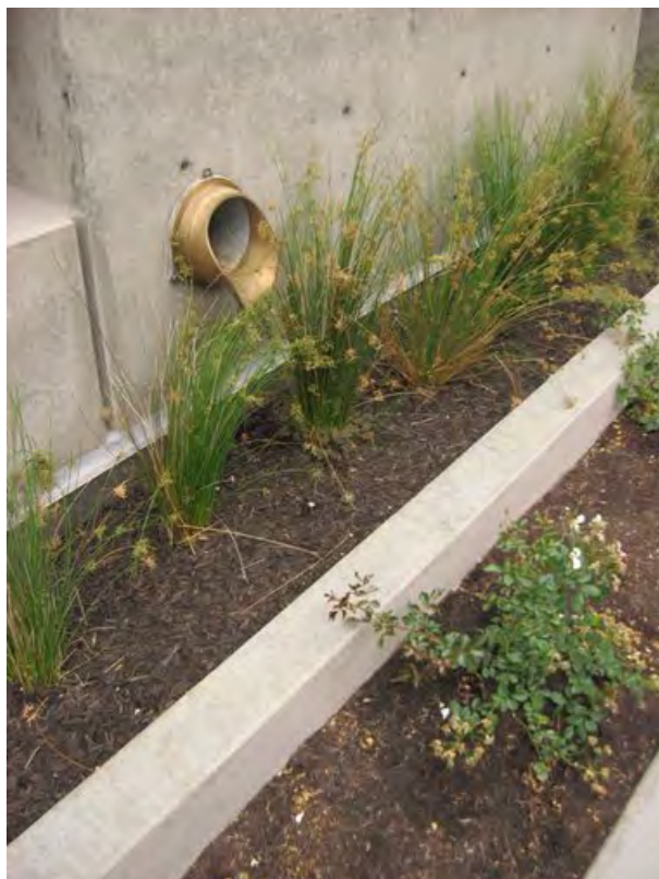
Figure 9. Disconnected downspout discharging to planter box.
