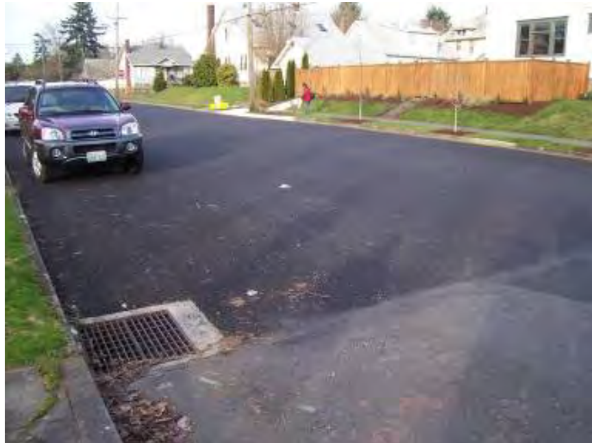
Figure 37. Pervious asphalt street in residential neighborhood in Portland Oregon. Source: Cahill Associates
