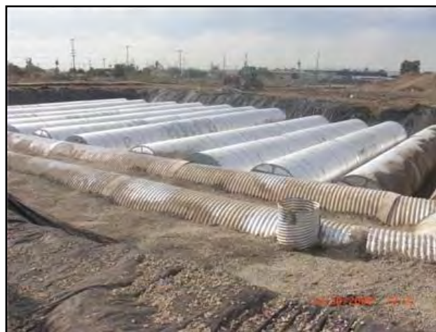
Underground Infiltration Units Lowe's, Pacoima
