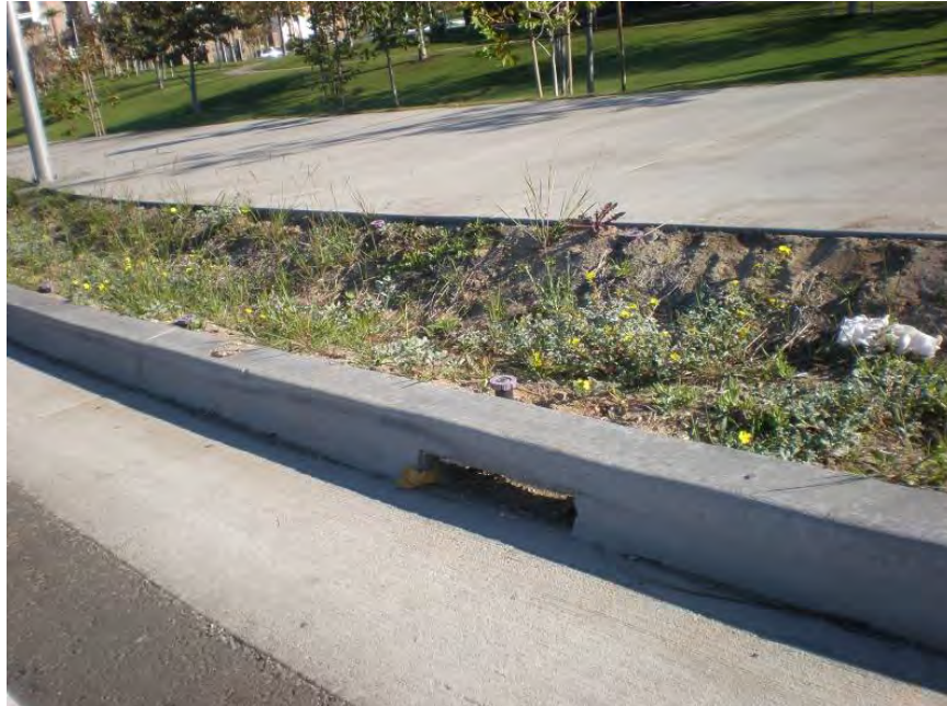
Figure 75. A vegetated swale with curb cuts in Playa Vista, California. Source: Keith Linker
