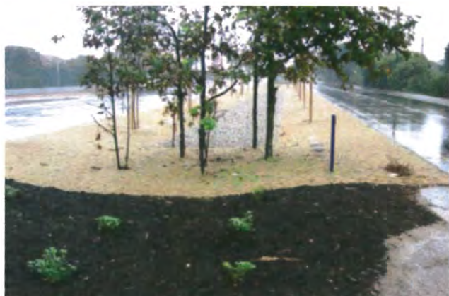
The Imperial Highway Greenway is an example of how roadways and rights-of-way can be converted into Green Solutions that naturally capture, filter and treat polluted runoff. Design and construction by PSOMAS.
