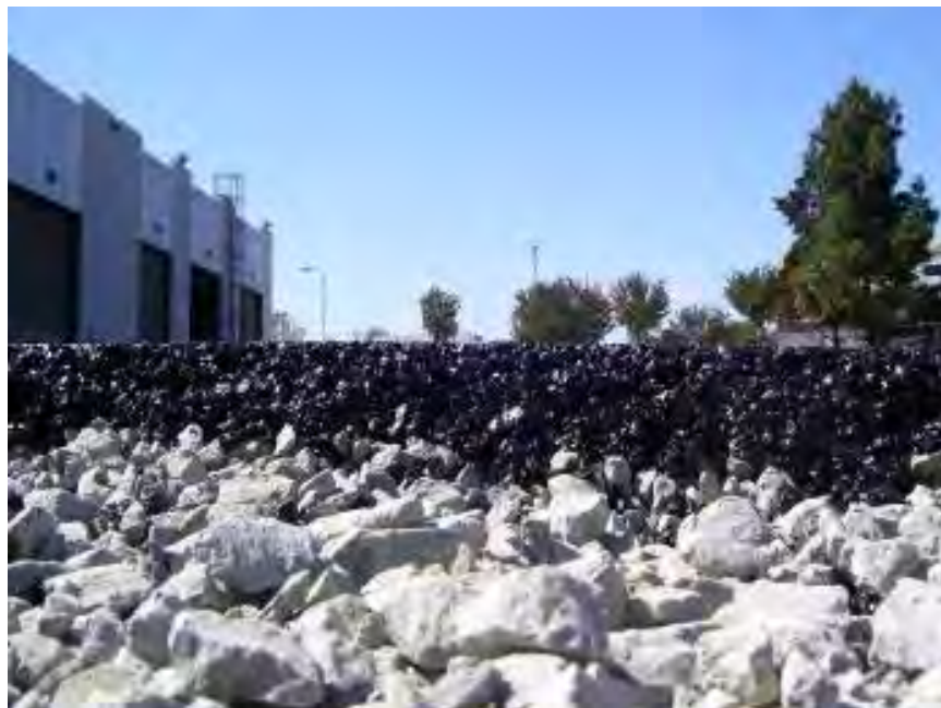
Figure 41. Close-up showing pervious asphalt pavement atop a stone infiltration/storage bed at the San Diego County Operations Center in Kearny Mesa, CA.
